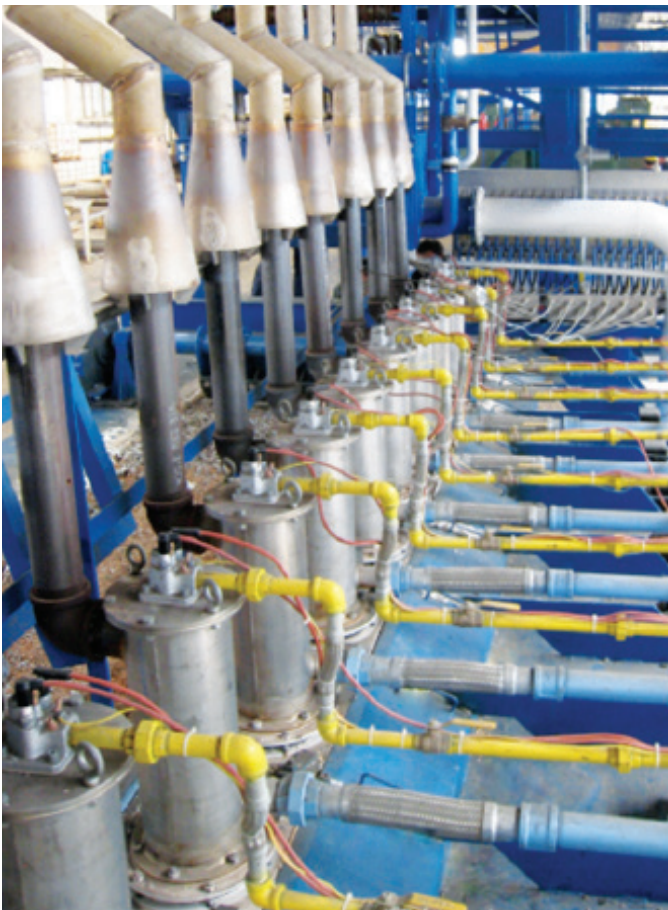
The latest Mk4 advanced recuperative burners on QED immersion burner galvaniser
